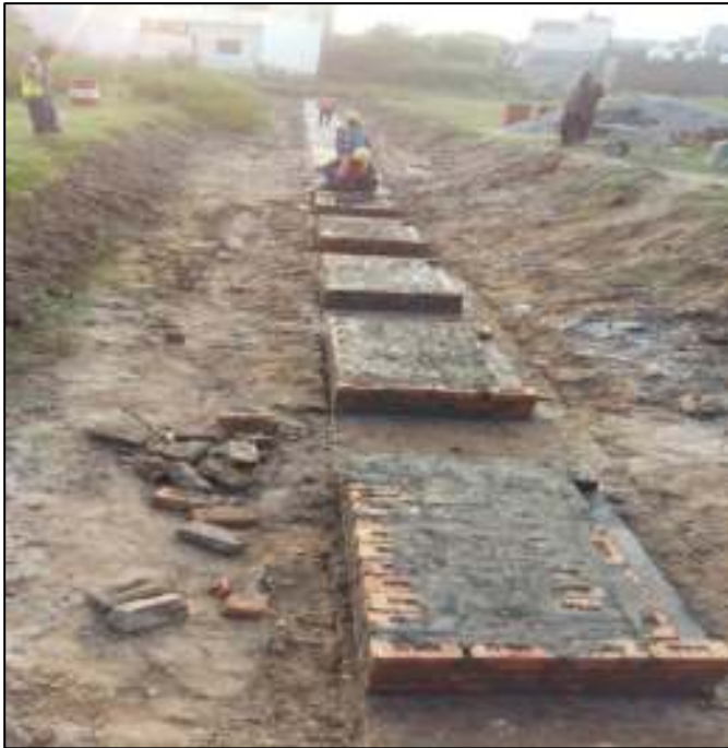
Picture 51: Brick Work & RCC Footing of Columns of Boundary wall of Pumping Station
