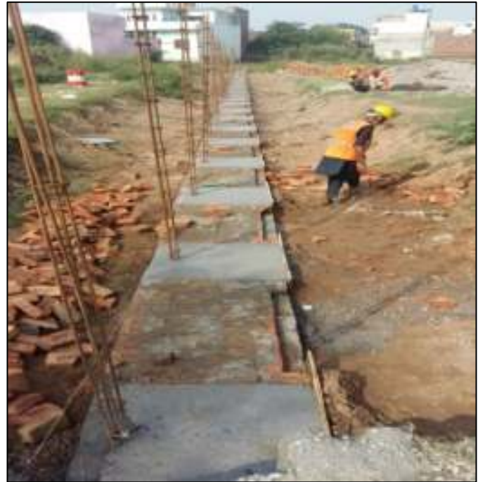
Picture 52: Brick Work & RCC Footing of Columns of Boundary wall of Pumping Station
