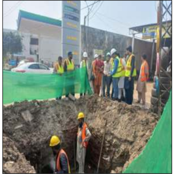
Picture 54: Conduits laying is in progress near Technical College Site 2 Marala Road Sialkot during ADB visit
