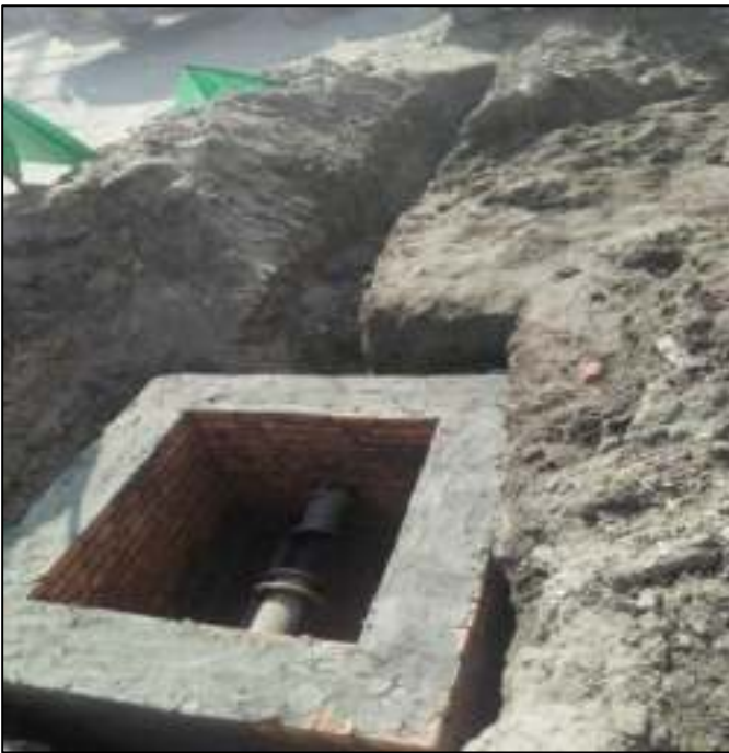
Picture 55: Gate Valve Chamber on Defence Road
